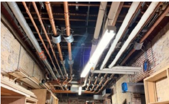
New mechanical systems
